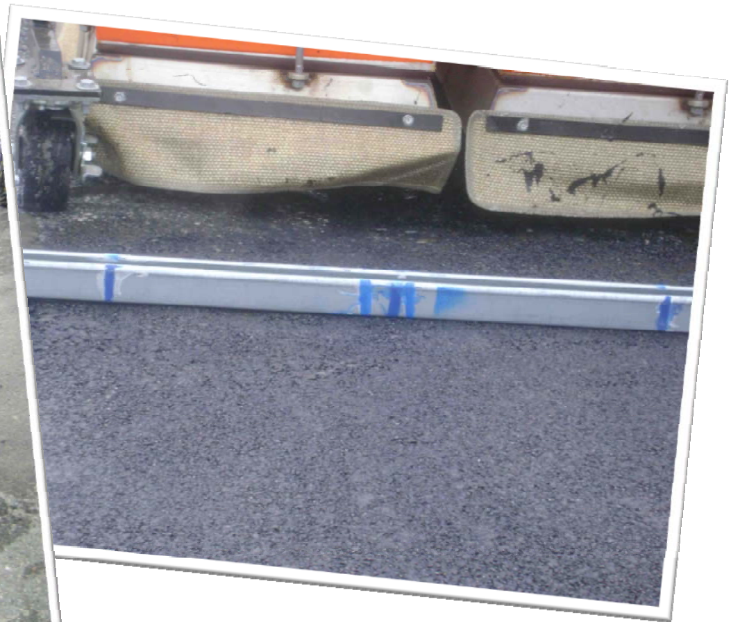
Level Check across crack
