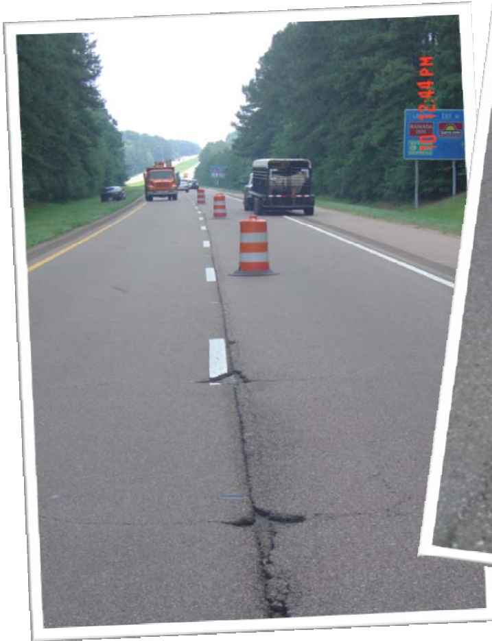
Typical failed joint, Mississippi
