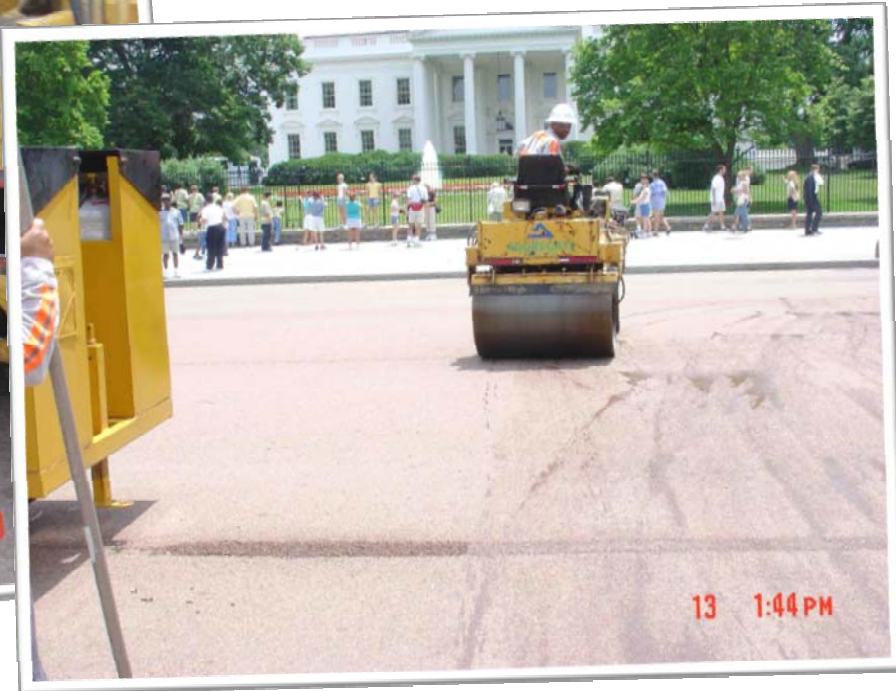
Compaction occurred close behind heater
